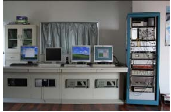
Figure 13-75. The control room of the Shanghai SLR station. The new pico-event timer (NPET) from Czech Technical University is shown in the middle of the rack; the timer was received in July 2009 and has a timing precision of 0.8ps.
