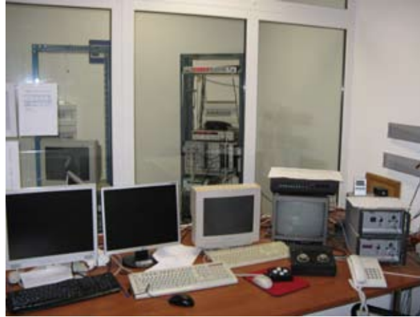
Figure 13-10. Station control room.
