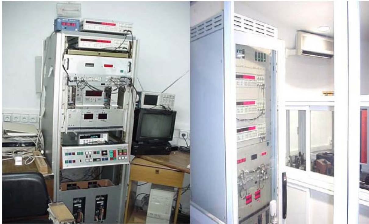
Figure 4: Timing devices in the control rack before and after the station refurbishment.
