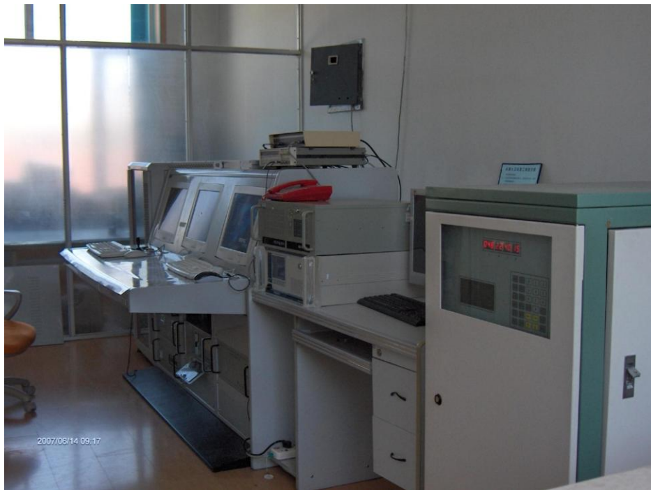
Figure 3. Changchun SLR & LTT Control Room
