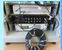
Fig.6 30m cable added to A033-B
