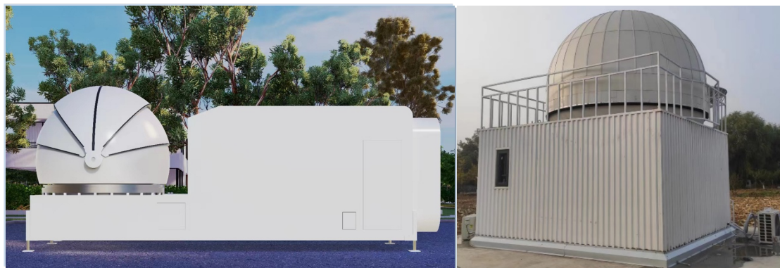
Figure 7. Two dedicated ground stations are under construction in China. A removable one is built in Xi'an (Left), and another fixed one is in Beijing (Right).
