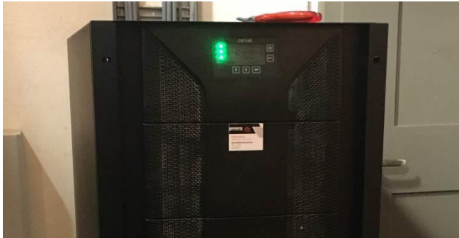
UPS 230VAC for entire station
